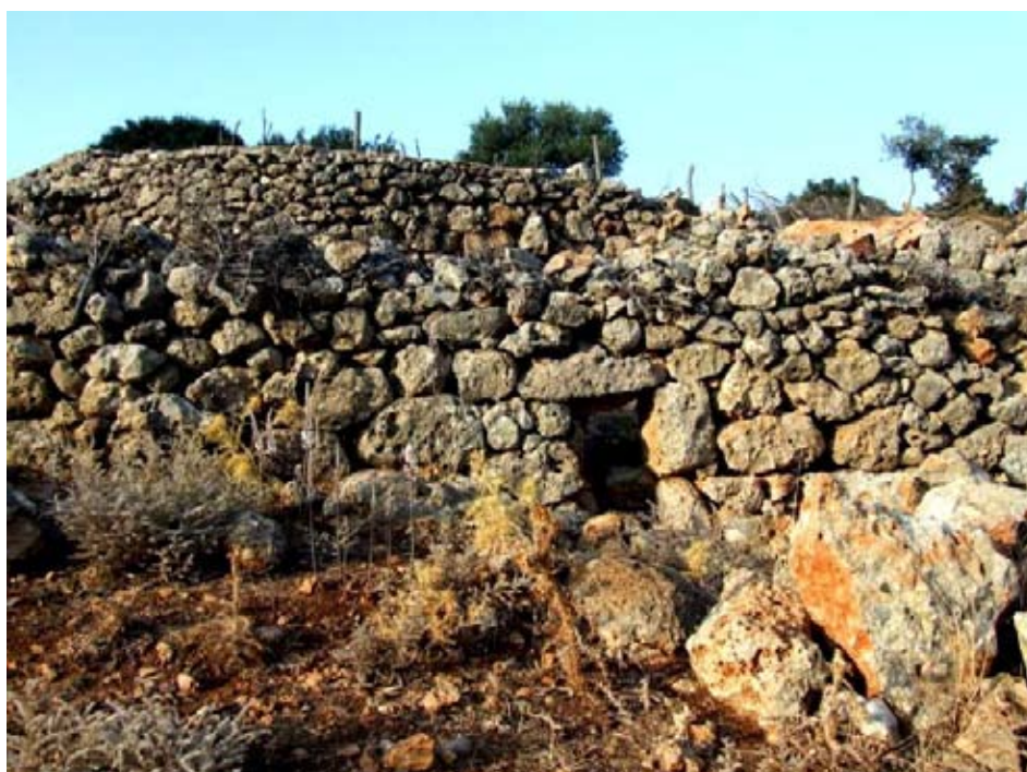
Figure 27: Mandra wall from outside with sewer opening. Kroustas area
